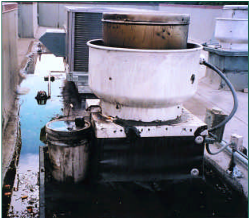
Photo 1: Grease spilling from a typical rooftop exhaust fan that does not have proper grease containment product in place
