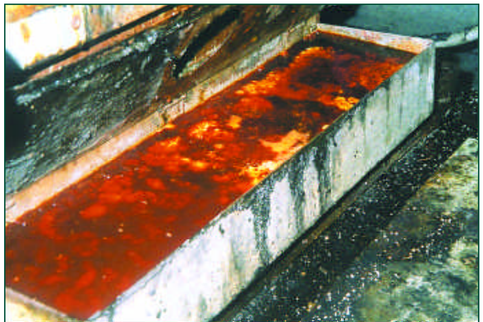
Photo 5: A collection box full of grease that is about to overflow.
