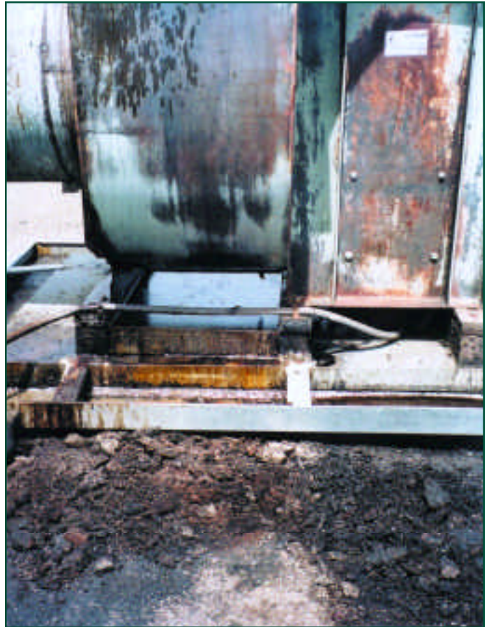
Photo 3: Roof damage caused by installing the improper grease containment product.
